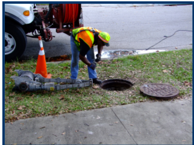
A TV camera is pulled through the newly lined sewers to assure high quality work.
