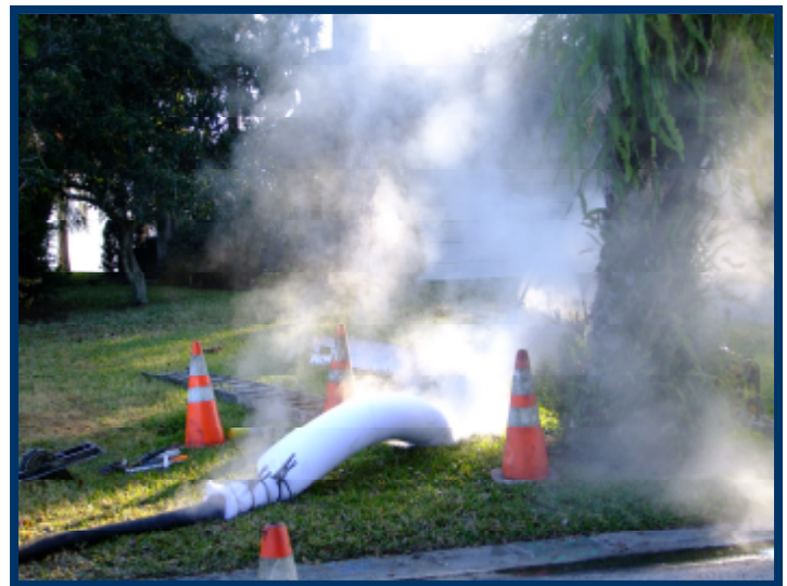
Steam is applied to the lining material within the old sewer pipe. The steam inflates the liner against the interior of the old pipe and the resin within the liner is activated by heat to form a new pipe inside the old one. All this is done without digging and is called "trenchless technology".
