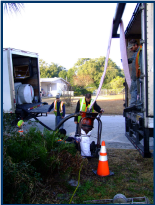
The pipe liners are inserted into the old sewer pipe using an inversion method.
