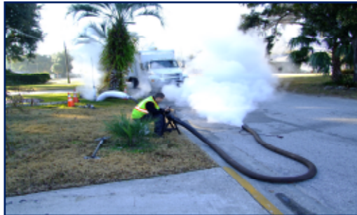
Crews use steam to activate the liner resin thus creating a new "pipe within a pipe."
