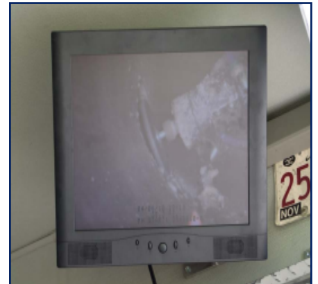
A robot cutter is used to remove a lining "coupon" to restore sewer service to every customer. It is guided using a closed circuit television (CCTV).
