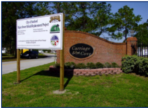
A sign informs the public that Federal "Stimulus" funds are being used for the project.
